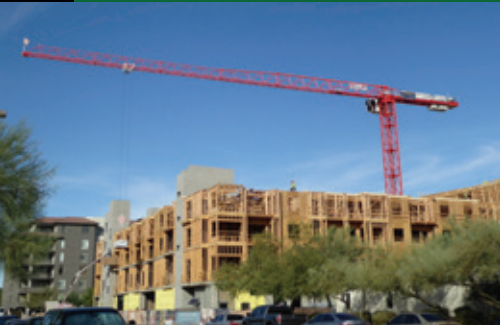
Compass Equipment provided a Wolff 6031.12 for the Overture Kierland project in Phoenix, AZ.
