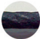
Lubricating covering broken wires making inspection impossible
