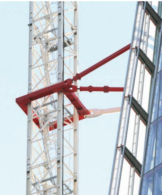
LEFT: Typical European-designed tie-in support with no access platforms
