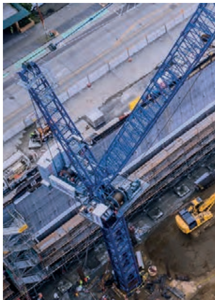
Top view of the wide hoisting winch platform in front of the Comansa LCL700 turntable
